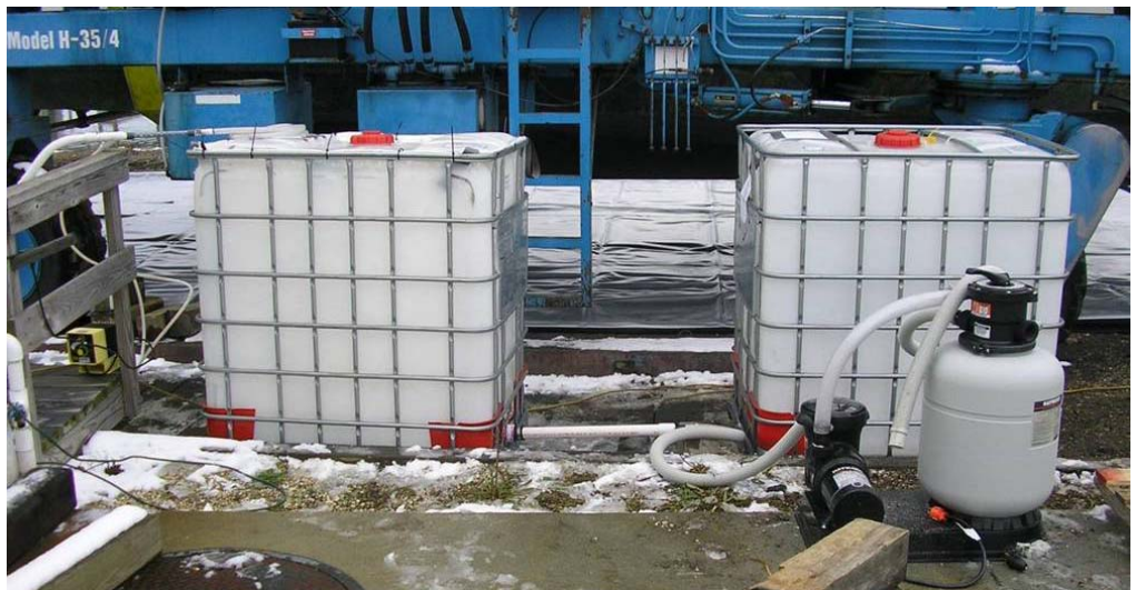
The complete wash wastewater treatment system
